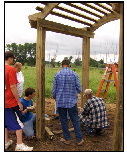
Eagle Scout Austin Reuter built a pergola along the hiking trail at the Hurstville Interpretive Center.
